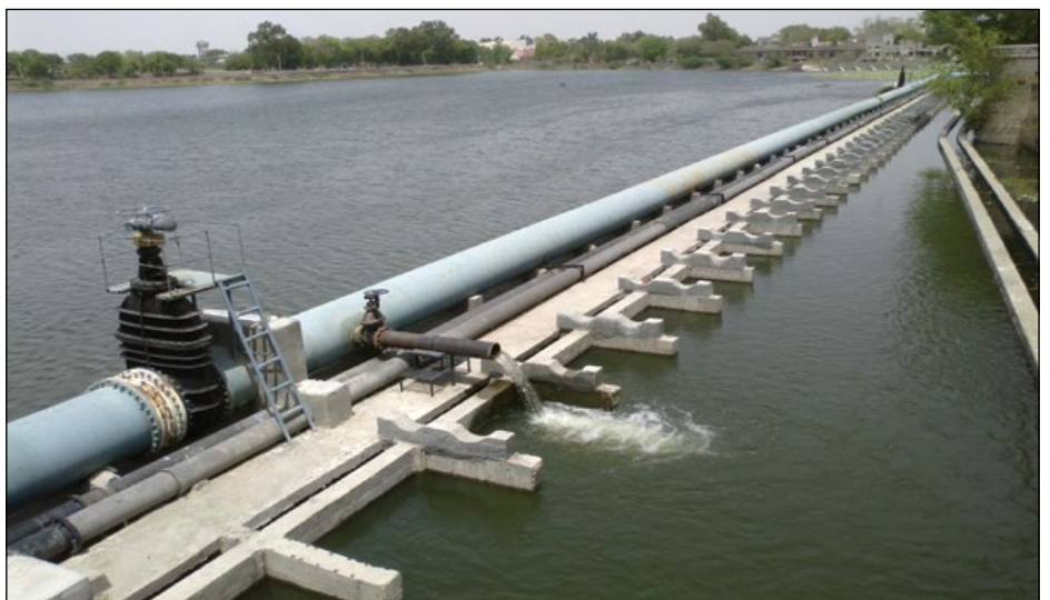
Water Supply Pipeline, Pali, Rajasthan
