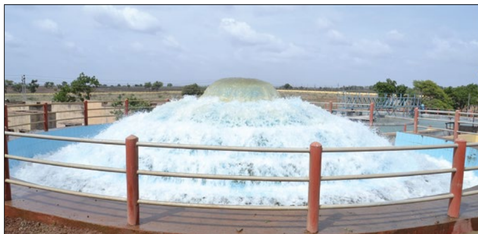
68 MLD Water Treatment Plant, Hubli-Dharwad, Karnataka
