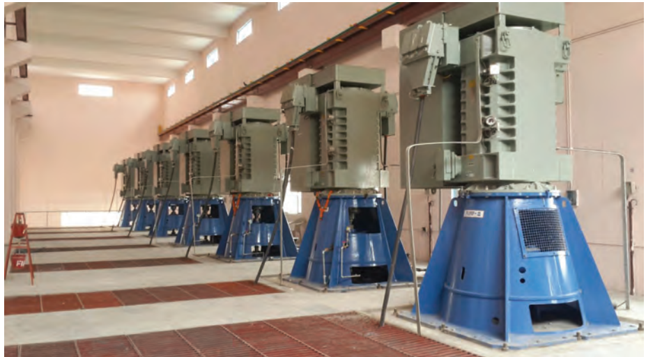
Sauni Phase 1 Pumping Station, Gujarat
