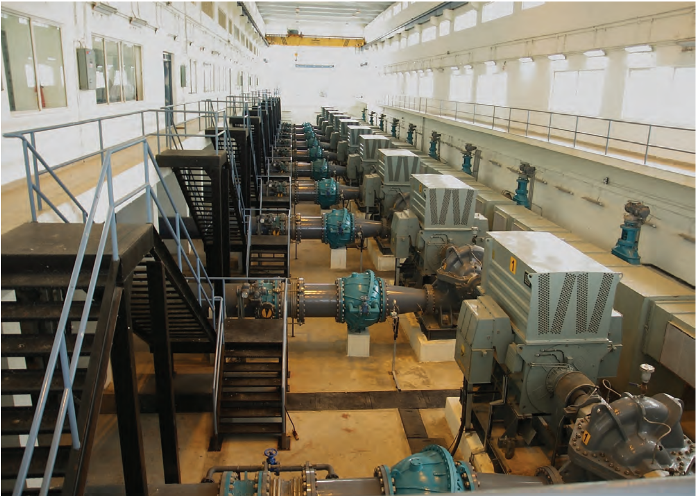
500 MLD Water Pumping Station, Bangalore
