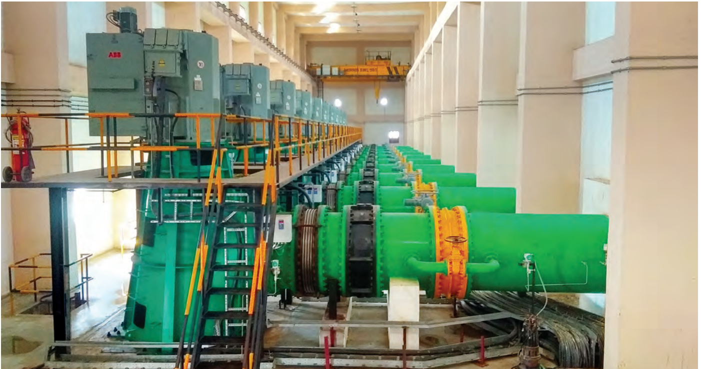
2587 MLD Pumping Station for SAUNI Yojana Phase-1, Gujarat
