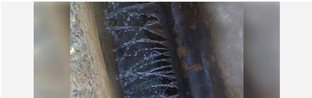
Damaged Supply Line in Bengaluru, India
