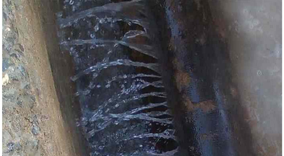
Damaged supply line in Bengaluru
