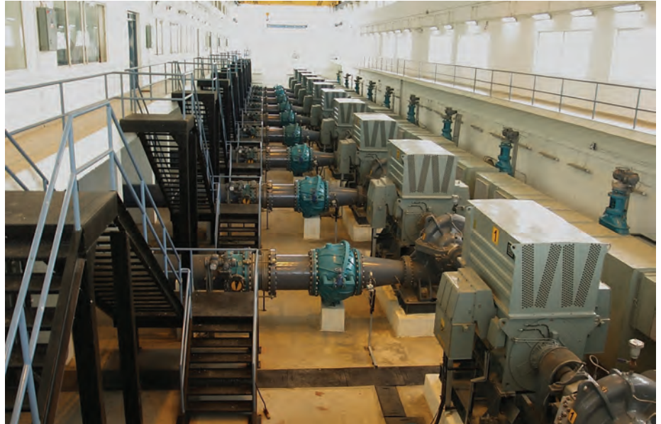
500 MLD Water Pumping Station, Bangalore
