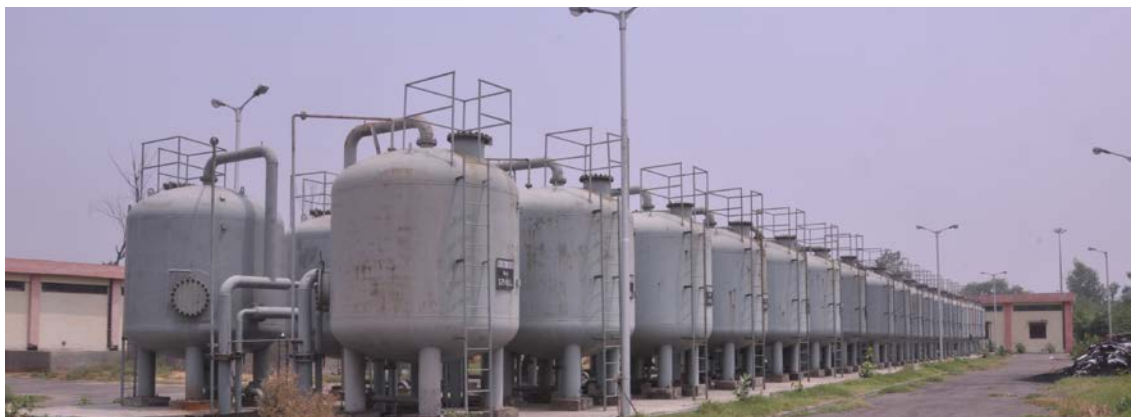
Activated Carbon Filter at CETP Naraina, Delhi
