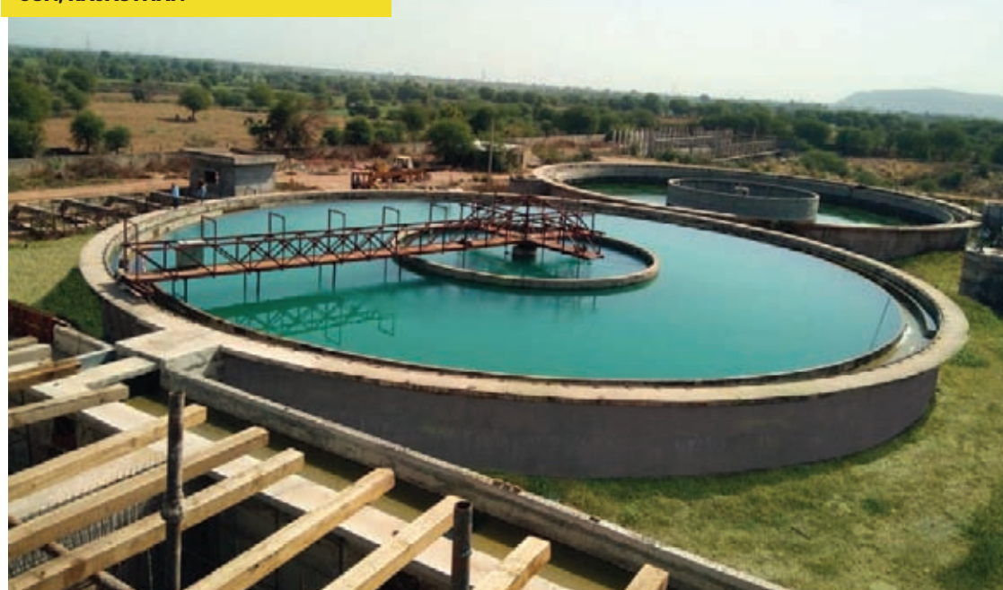
146 MLD WATER TREATMENT PLANT, CSN, RAJASTHAN
