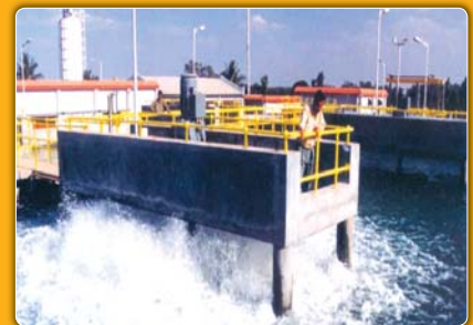
Yelahanka Primary/Tertiary Sewage Plant - Created the first of its kind sewage treatment plant for the reuse of municipal wastewater in India
