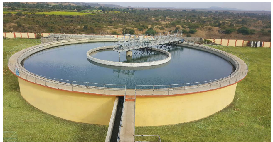
19 MLD Water Treatment Plant, Gagreen, Rajasthan
