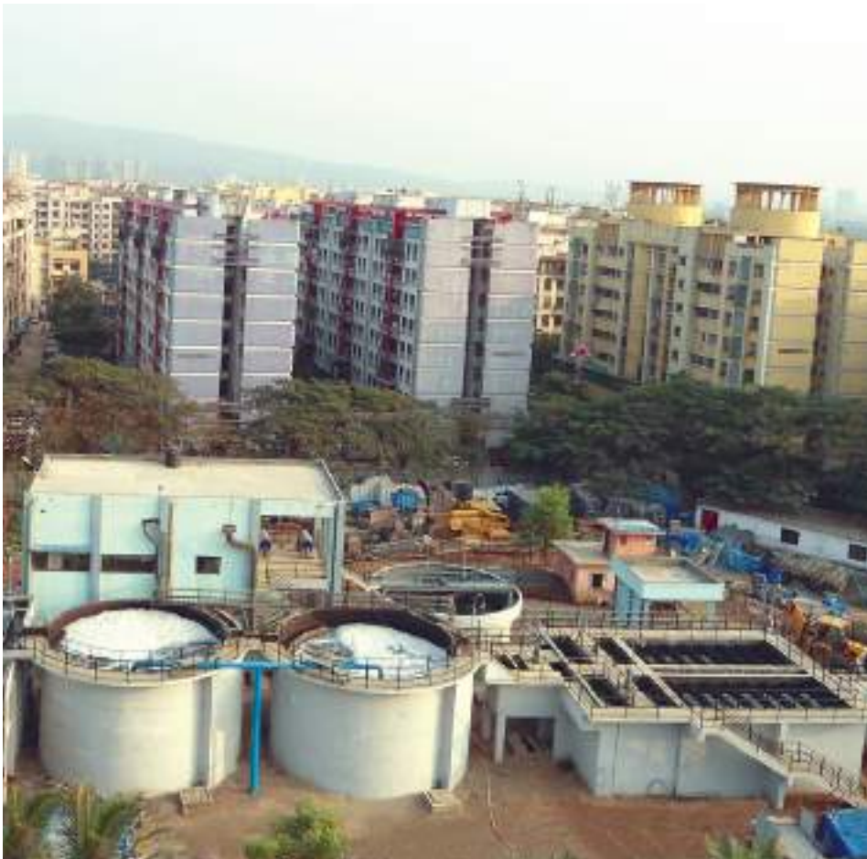
11 MLD Decentralised Sewage Treatment Plant at Mira Bhayander
