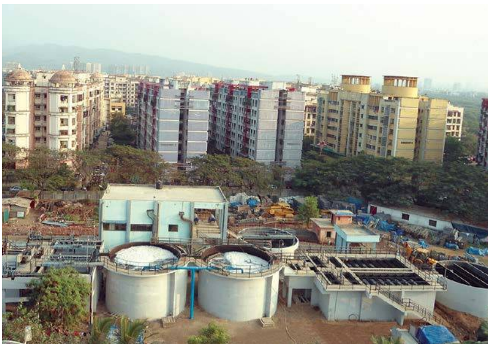
11 MLD Decentralized Sewerage Treatment Plant at Mira Bhayandar
