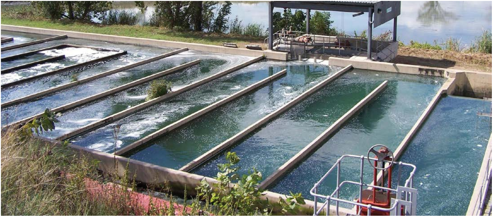
Chlorine Contact Tank at Mira Bhayandar
