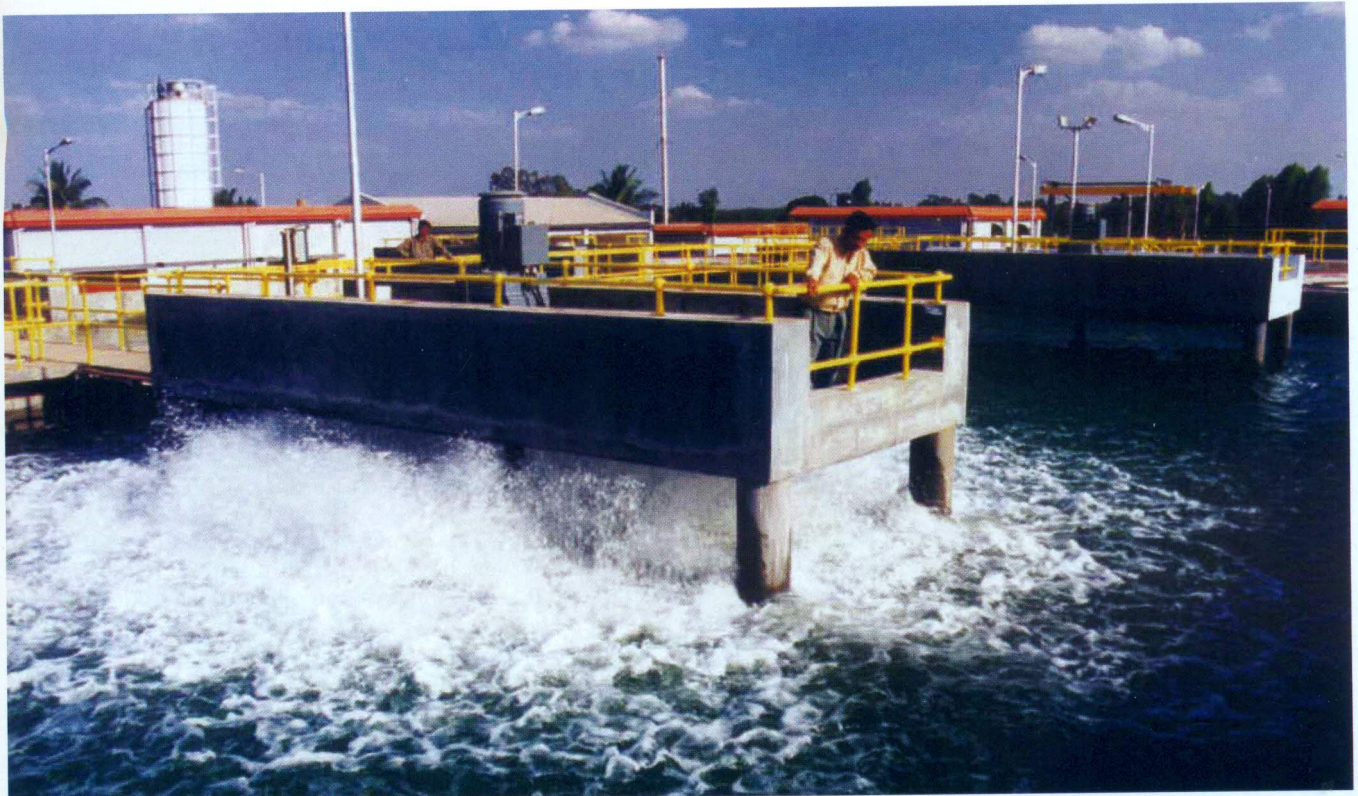
Tertiary Treatment Plant, Bangalore
