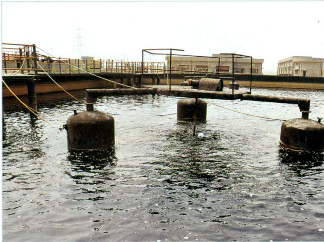
Demographic trends and increasing urbanisation are the two key factors for increase in wastewater
