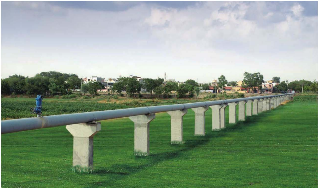
Bisalpur-Jaipur water supply pipeline.
