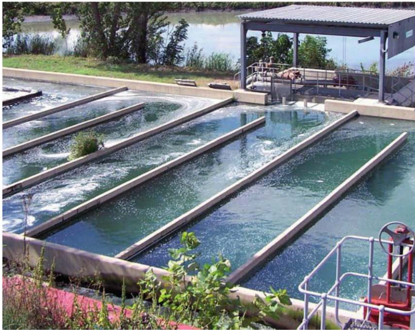
A water treatment plant at Pokhran in Rajasthan.
