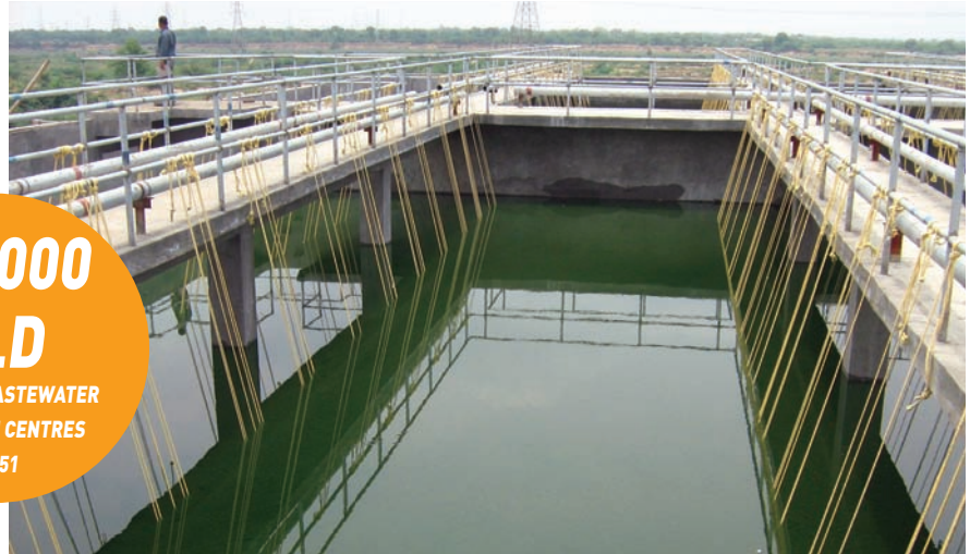
Storage tanks at a wastewater plant
