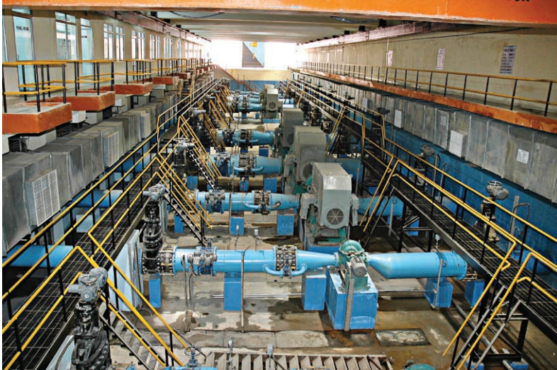
Jaipur Water Pumping Station
