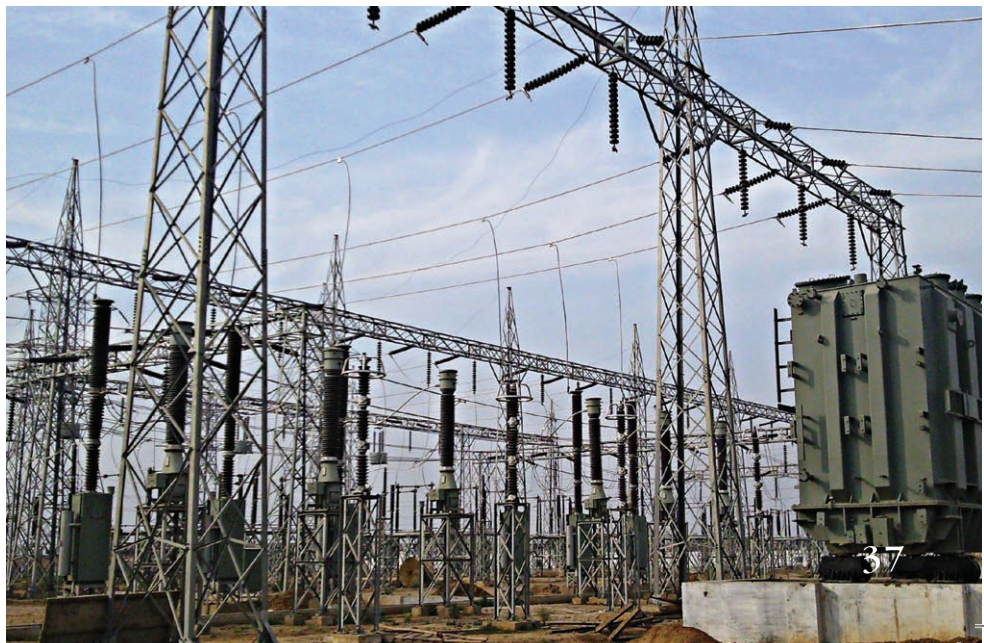
Power Substation at Ramgarh, Rajasthan
