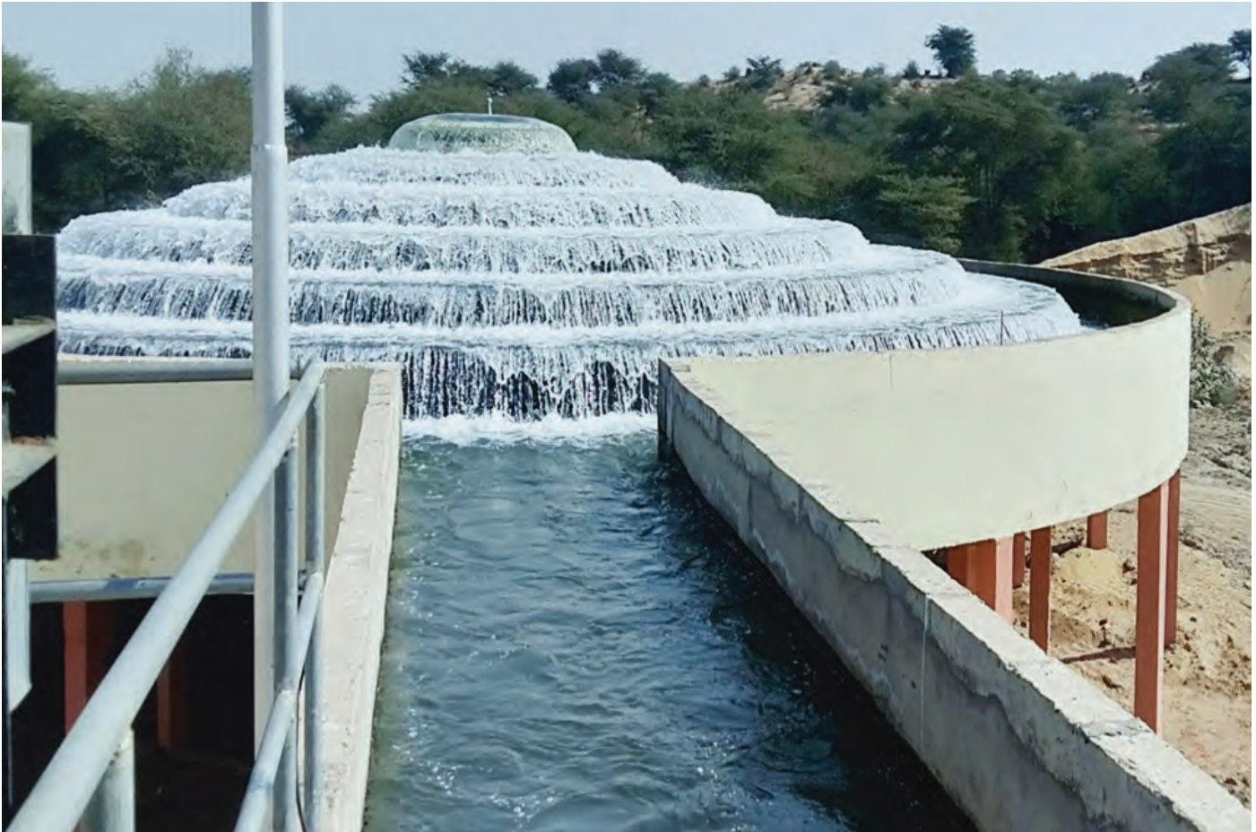
Water Treatment Plant, Rajasthan
