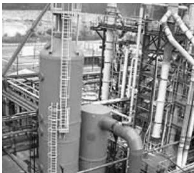
Gas Cleaning Plant
