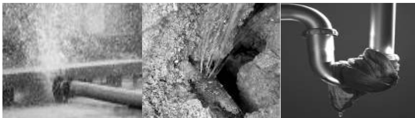
Fig 2.6 Pipe line leaks
