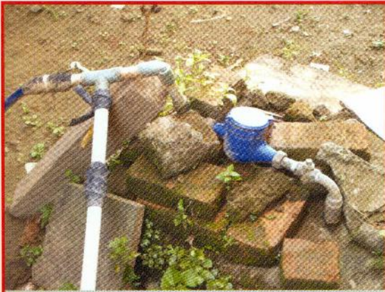
Customers aware of poor service caused by water losses will report defective connections.
