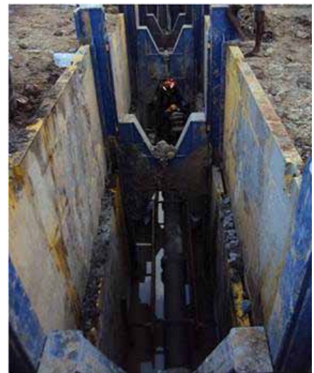
Photograph shows use of imported shoring material from SBH, Germany during laying of pipeline for the safety of workmen due to unstable strata
