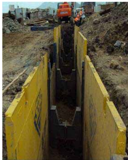
Photograph shows removal of shoring material after laying of pipeline is over
