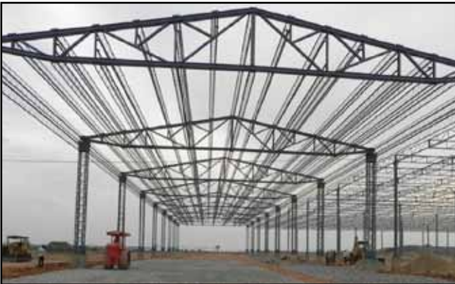
Tipping Area – Pad Work is in Progress. Expected to be completed by 06.02.2011 Machine Erection in this Area can start from 21.02.2011
