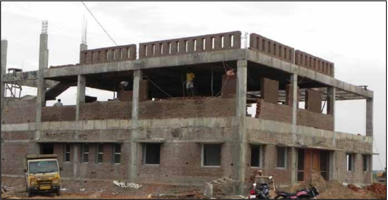
Admin Building: Internal Plastering for Ground Floor Over, First Floor Brick Work is in Progress.
