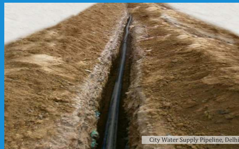
Bisalpur-Jaipur Water Supply Pipeline, Rajasthan
