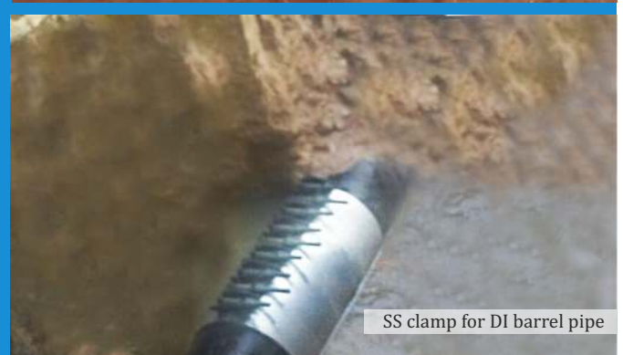
Damaged supply line
