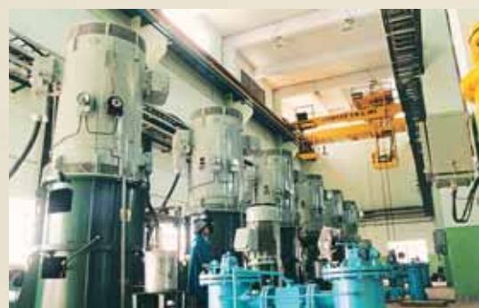
Water Pumping Station, Dharnasar in Rajasthan
